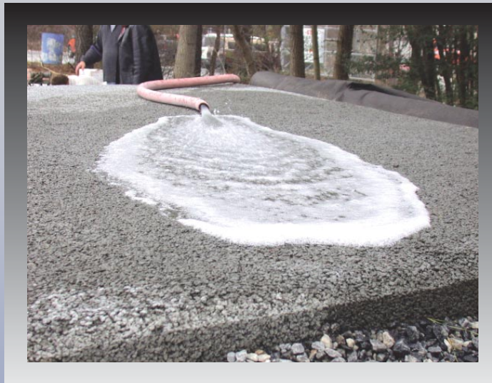
Fig. 1. Pervious concrete allows water to flow through it, allowing recharge of groundwater and reducing the need for storm water retention areas. (IMG13626)
