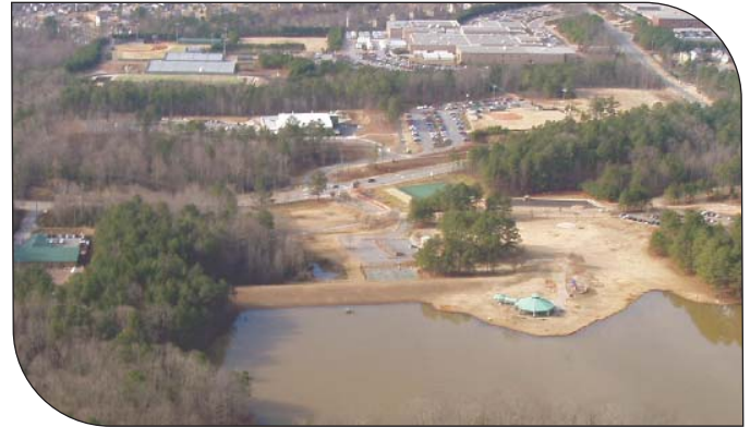
Aerial view of the Y-17 dam and downstream reach prior to rehabilitation.
