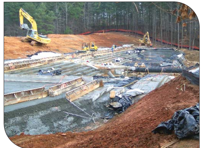
Completion of the RCC stilling basin and construction of the RCC spillway steps and sidewalls.
