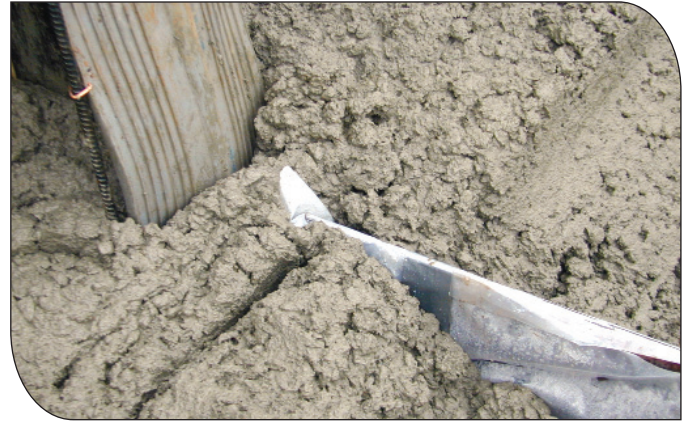
A close up view of water stop, conventional concrete for upstream facing, and contraction joint materials
