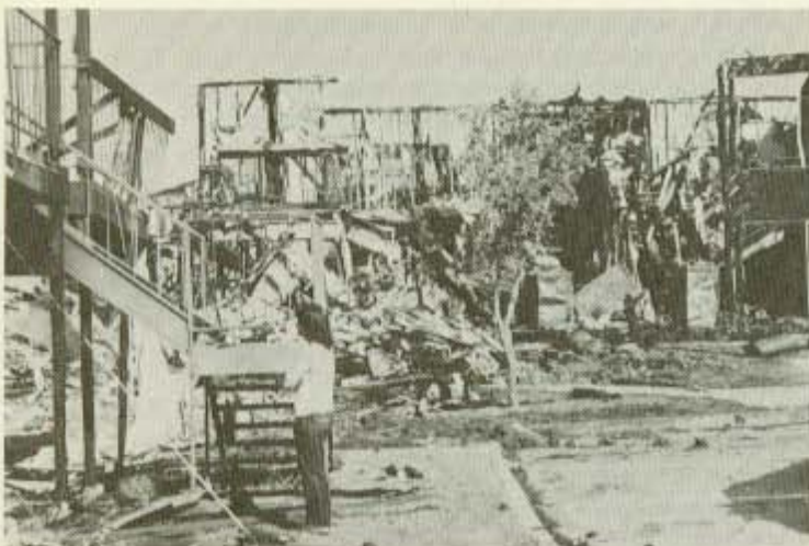
This is the charred wreckage of a five-alarm fire that destroyed 100 units in 10 buildings of two fashionable apartment complexes. Fire-resistant construction can help prevent this destruction. (Photo by David G. Baker)
