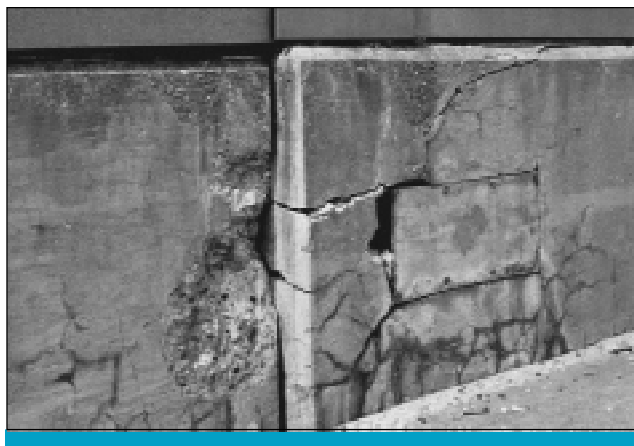
Fig. 1. ASR has led to damage and relative displacement of this parapet wall.
