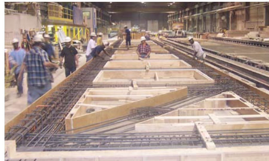
Fig. 17. This production photo was taken at Hanson Structural Precast—Midwest facility during manufacture of open-space truss.
