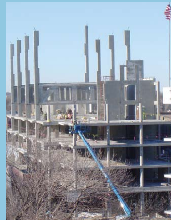
This precast concrete erection photo illustrates the modular stacking method of assembly during construction of Cobalt condominiums.
