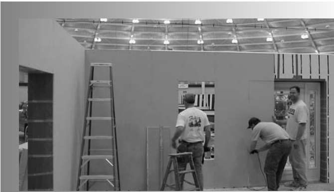
Top: Volunteers are busy constructing the ICF Habitat for Humanity home inside the Joyce Athletic Center in advance of the show.
