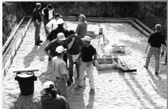
(Bottom) An eager crew of volunteers prepares for the arrival of concrete to be placed in the footings.
