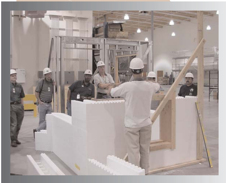
UBC Journeymen Instructors listen to Ivan Panushev of Building Works Inc., discuss the finer points of ICF wall construction.
