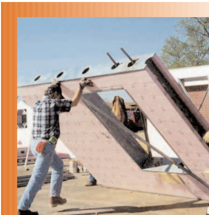
ICF wall panels can be pre-assembled and set into place by one worker, as shown in this photo of a construction site in Lubbock.
