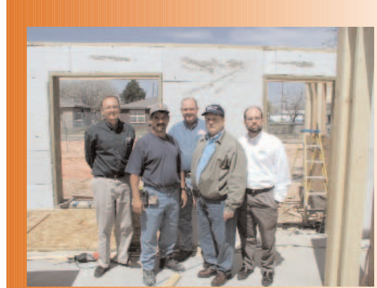
Brad Reed and others take a moment to pose for the camera in front of an Eco-Block ICF wall system under construction in Lubbock.
