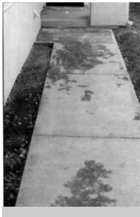
Fig. 1 Severe discoloration of concrete flatwork is usually caused by a combination of factors.
