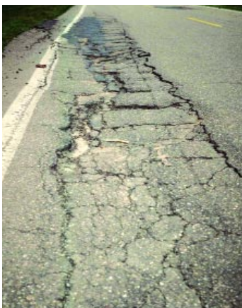
Base Failure Cracking
