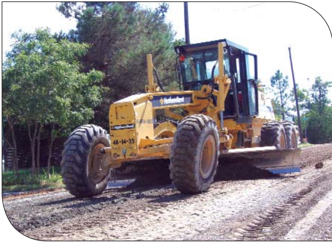
Motorgrader operator re-shapes the street after adding cement to the existing pulverized material.
