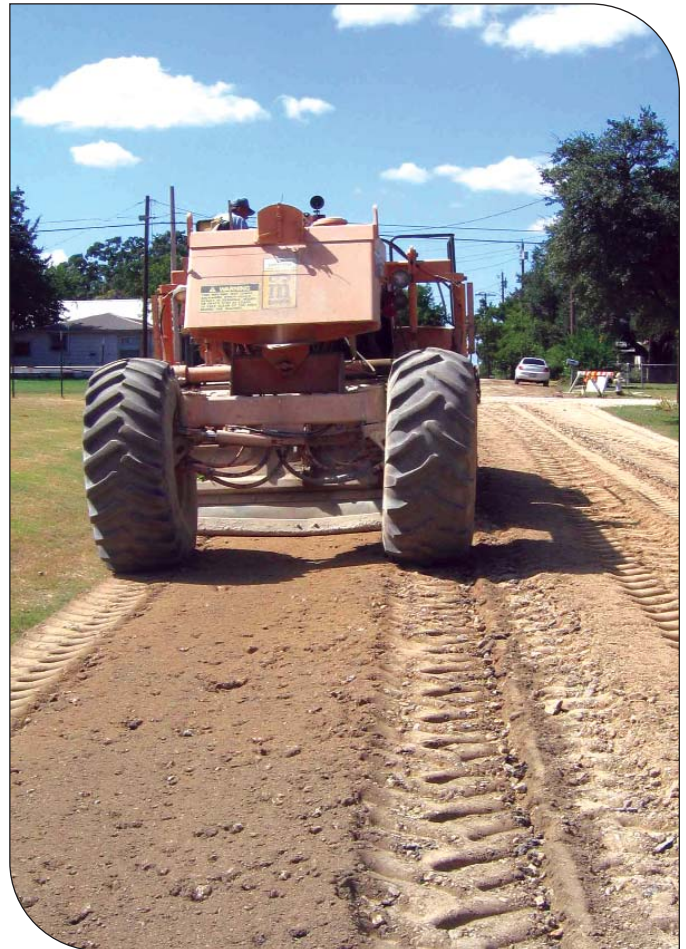
Reclaimer pulverizes the existing street. One or two passes usually achieves gradation requirements.
