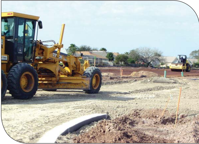
CTB is spread on the prepared subgrade where it is then graded, compacted, and cured.
