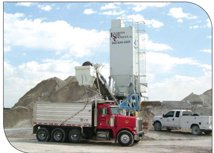
CTB is mixed in an ARAN pugmill and transported to the roadway in dump trucks.
