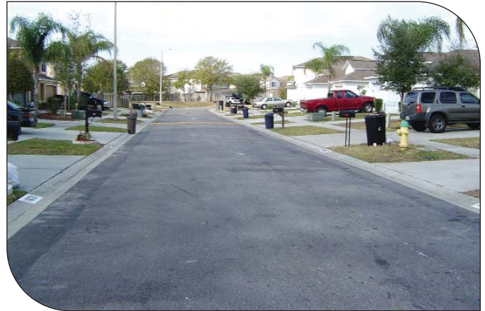
This street was constructed with CTB over eight years ago and shows no signs of distress.
