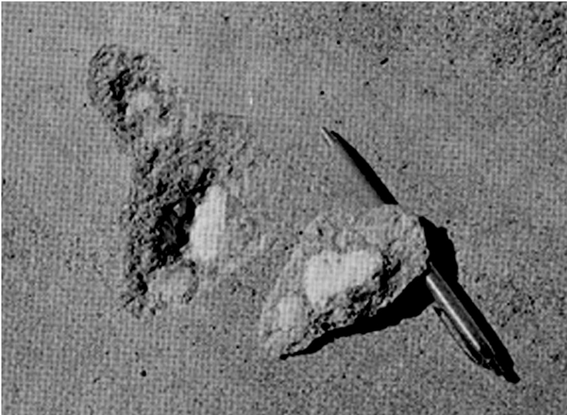
Figure 8. A popout is a small fragment of concrete surface that has broken away due to internal pressure, leaving a shallow, typically conical, depression. (0113)
