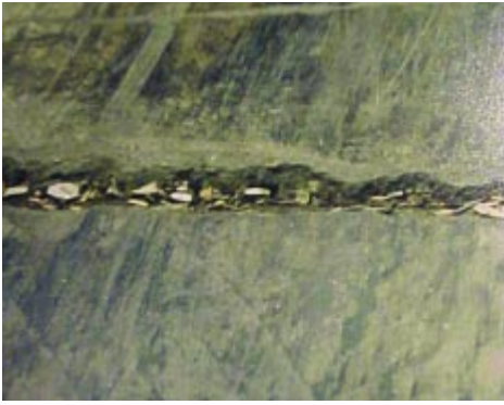
Fig. 22. A common form of impact overload occurs at slab edges of joints on vehicular traffic surfaces. (70151)
