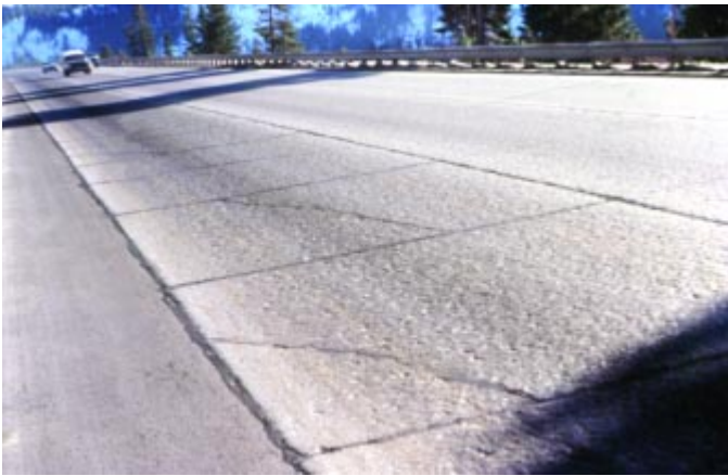
Fig 16. Tire chains and studded snow tires can cause considerable wear to concrete surfaces. (70156)
