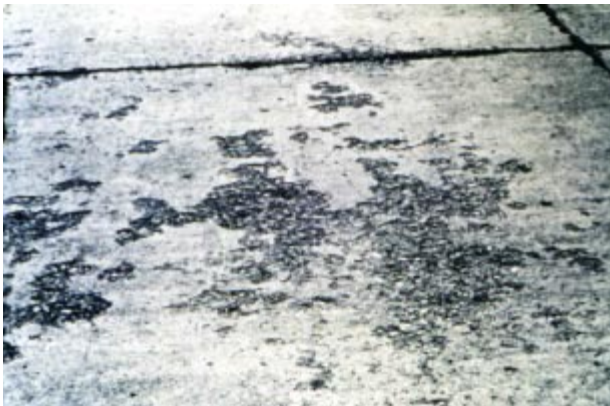
Fig 6. Freeze-thaw cycles can cause scaling of concrete surfaces. (A5273)
