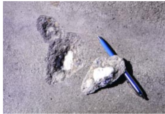
Fig. 8. Some aggregates absorb water and, upon freezing, expand to produce a popout. (0113)
