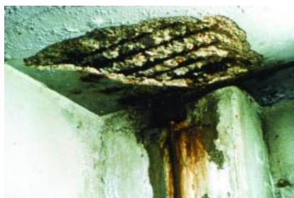
Fig. 1. Corrosion of reinforcing steel is the most common cause of concrete deterioration. (46080)
