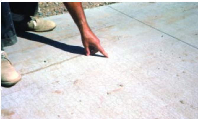
Fig. 30. Crazing typically does not penetrate much below the surface and is usually a cosmetic problem only. (4099)
