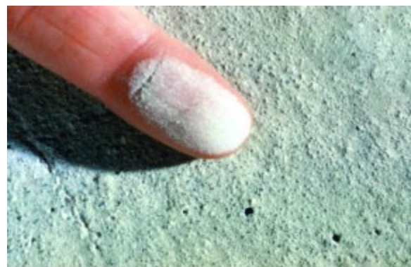
Fig. 28. Dusting is the development of a fine, powdery material that easily rubs off the surface of hardened concrete. (1297)
