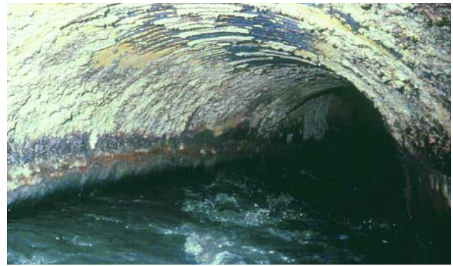
Fig. 11. Bacteria in sewage systems can produce sulfuric acid, which aggressively attacks concrete. (70149)
