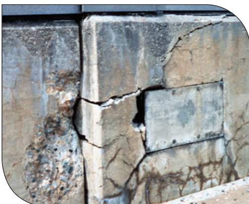
Figure 3. This parapet wall has been severely affected by ASR. Notice the cracking, joint closing, spalling of concrete surfaces, and lateral offset that have developed. (IMG12295)
