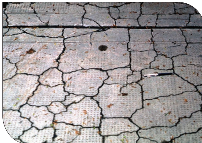
Figure 21. Map cracking pattern caused by ACR (IMG12982).
