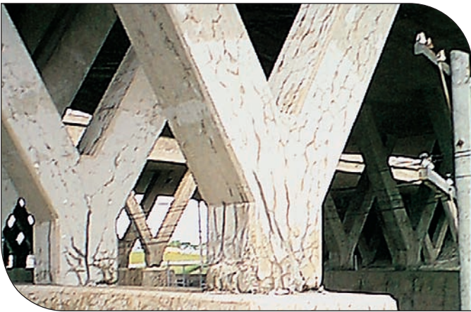
Figure 10. Cracking associated with stress directions. Predominant cracks are oriented longitudinally in this column. (IMG12421)
