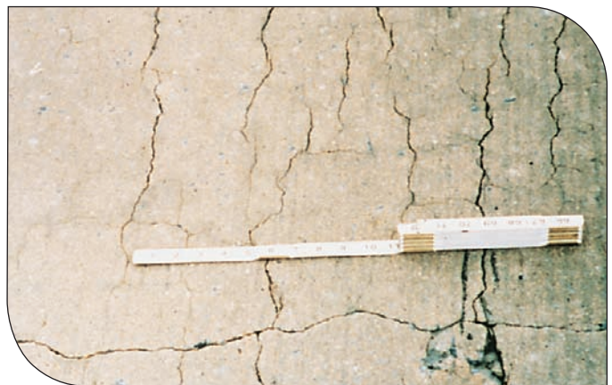
Figure 5. Close-up view of well developed cracking in a pavement, a typical pattern associated with ASR. The prominent cracks are in a longitudinal direction as there is less restraint to lateral expansion. (IMG13049)
