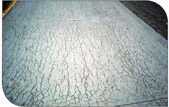
Figure 4. Longitudinal cracks induced by ASR in a concrete pavement. (IMG21371)
