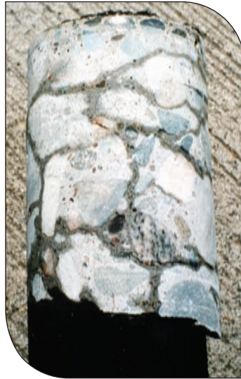
Figure 6. Cracks can be more easily seen when the concrete has been wetted and is starting to dry. (Stark 1991a). (IMG12986)
