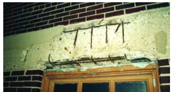
Fig. 5. Carbonation-induced corrosion often occurs on building facades with shallow concrete cover. (70157)
