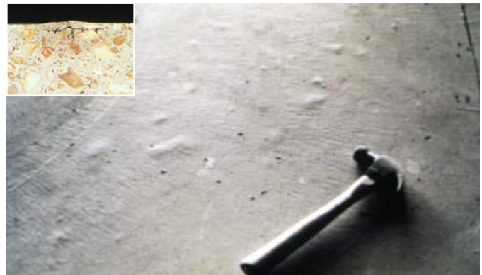
Fig. 27. Delaminations and blisters occur when air and bleed water become trapped under a prematurely closed (densified) mortar surface. (Photo courtesy of NRMCA.) (A5272, 49411)
