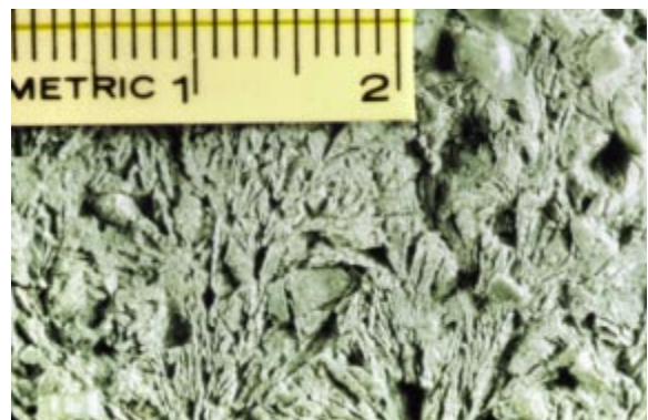
Fig. 9. Ice crystals often form in concrete that is frozen before it hardens. The disruption of the paste matrix by freezing can cause reduced strength gain and increased porosity. (44047)
