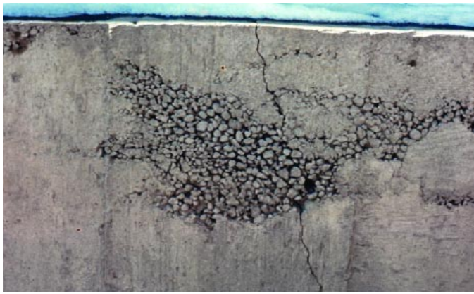
Fig. 25. Honeycomb occurs when mortar fails to fill the spaces between coarse aggregates. (70152)
