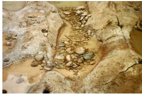
Fig 17. The abrasion of debris in rushing water can produce significant wear on concrete surfaces. (70150)
