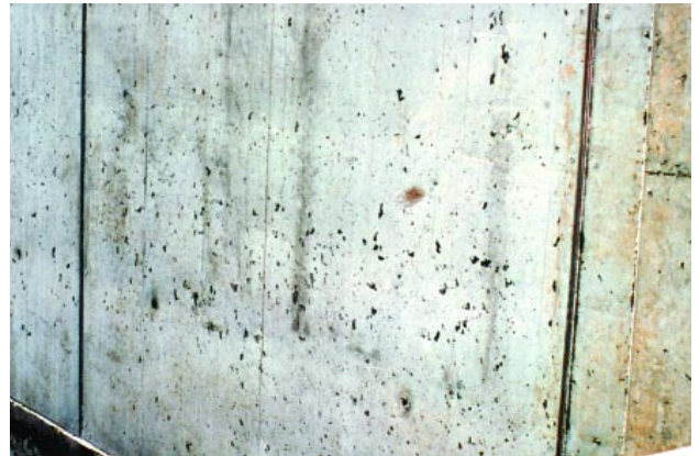
Fig. 24. Surface air voids, or bugholes, are small cavities of entrapped air bubbles in the surface of formed concrete. (70154)
