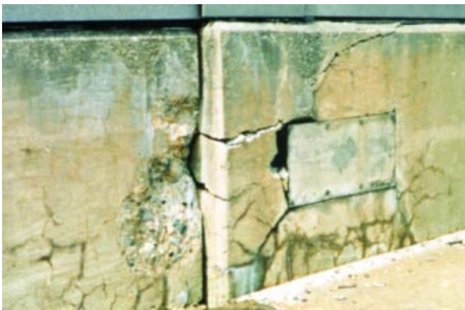
Fig. 14. Typical indicators of alkali-silica reactivity are map cracking and, in advanced cases, closed joints and spalled concrete surfaces. (56586)
