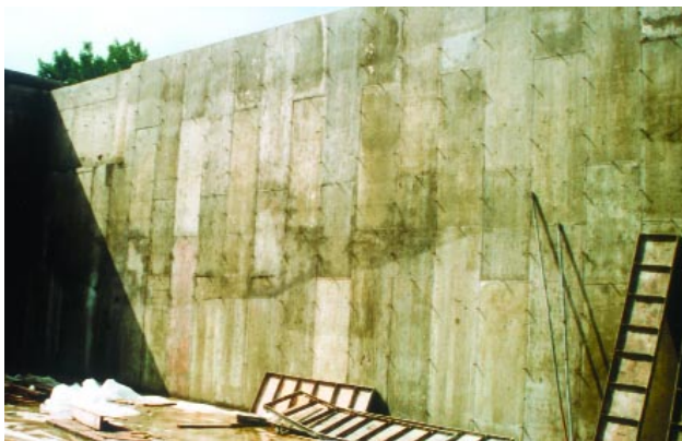
Fig. 26. Cold joints often result in visible lines where one layer of concrete had hardened before subsequent concrete was placed, as shown here in a sloping horizontal line. (70153)
