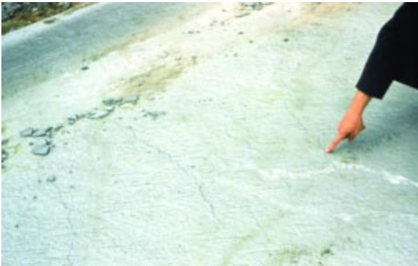
Fig. 20. Plastic shrinkage cracks can occur when water evaporates from the surface faster than it is replaced by bleedwater. (1311)
