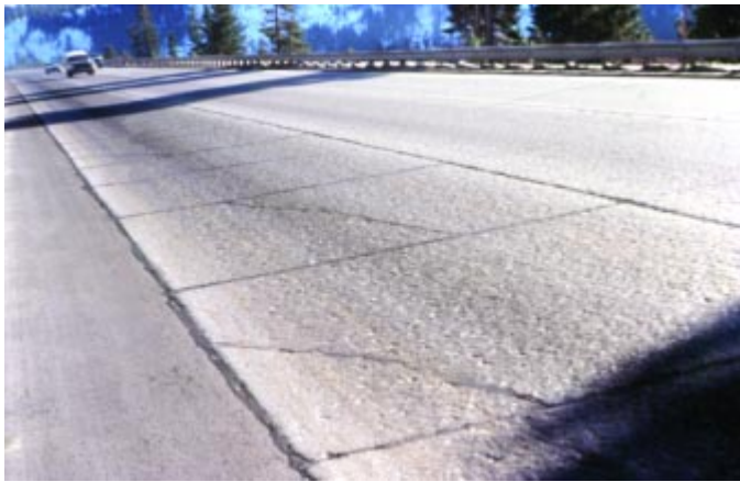
Fig 16. Tire chains and studded snow tires can cause considerable wear to concrete surfaces. (70156)
