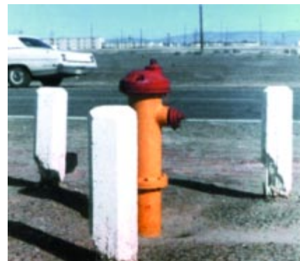
Fig 12. The bases of these concrete posts have suffered from sulfate attack. (66900)
