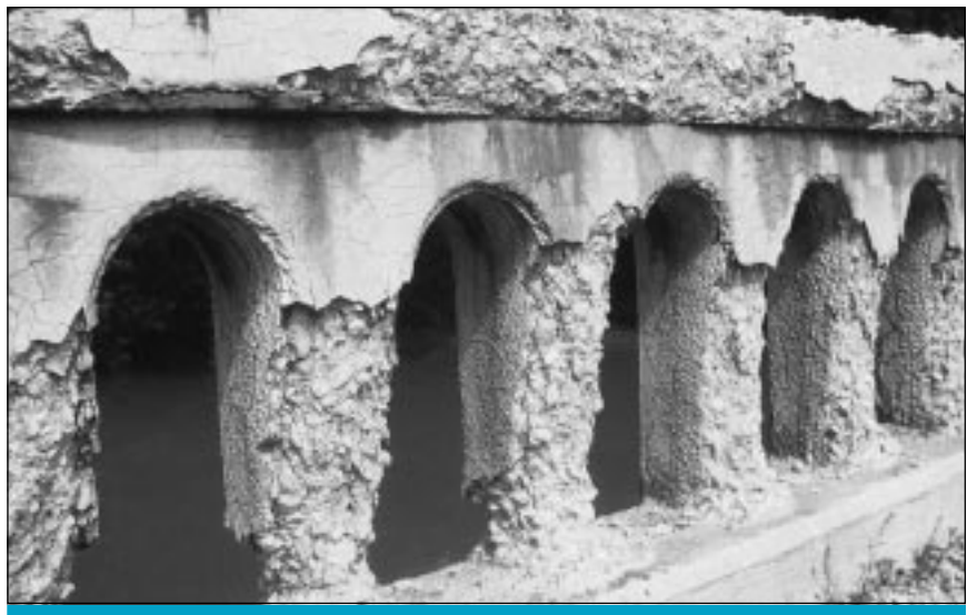
Figure 1. Freeze-thaw deterioration of non-air-entrained concrete railing. (S44517)
