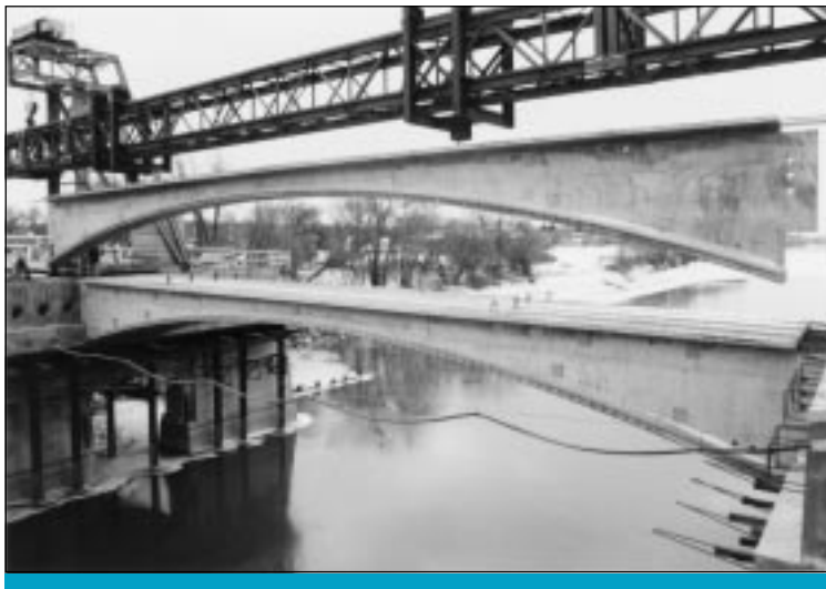
Figure 4. Precast sections made with concrete bar supports being placed at Norwood Bridge. Photo courtesy of Lafarge Canada Inc.-Winnipeg Precast and Thomas Young Productions (photographer).
