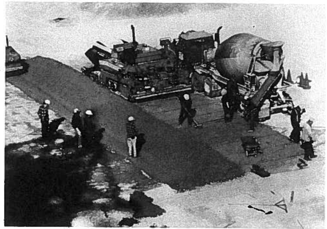
Fig. 11. U.S. Bureau of Reclamation/Portland Cement Association joint research project on bonding successive layers of roller-compacted concrete.
