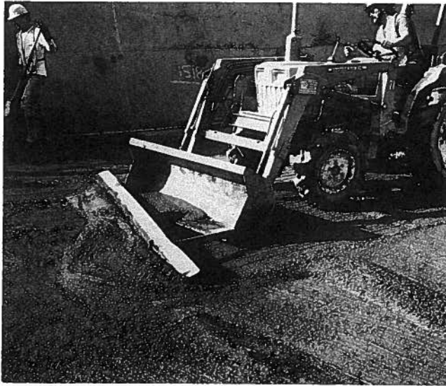
Fig. 10. Spreading mortar bedding layer onto RCC surface at Elk Creek Dam, Oregon (courtesy of U.S. Army Corps of Engineers, Portland, Oregon).
