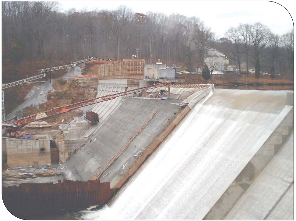
RCC nearing completion on the west section of spillway while the east section is operating. Note the RCC mixing plant and conveyor system in the background.
