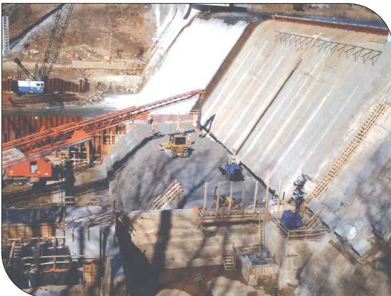
RCC placement on the east section of spillway while the west section is operating.
