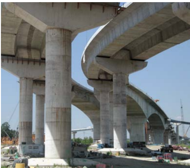
Figure 1. Mass concrete columns and footings for the James River Bridge. (Courtesy of Fred Parkinson, PB.)
