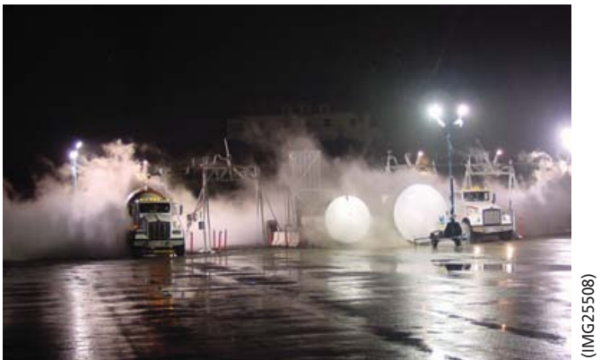
Figure 27. Five liquid nitrogen cooling stations were set up to provide a consistent flow of concrete.
