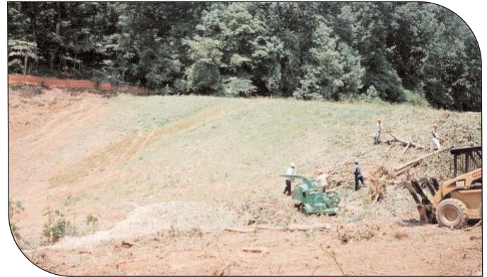
Y-14 Structure during the early stages of construction (clearing and grubbing in process)
