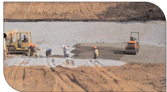
Placement of the first lift of RCC in the stilling basin area at the toe of the existing dam
